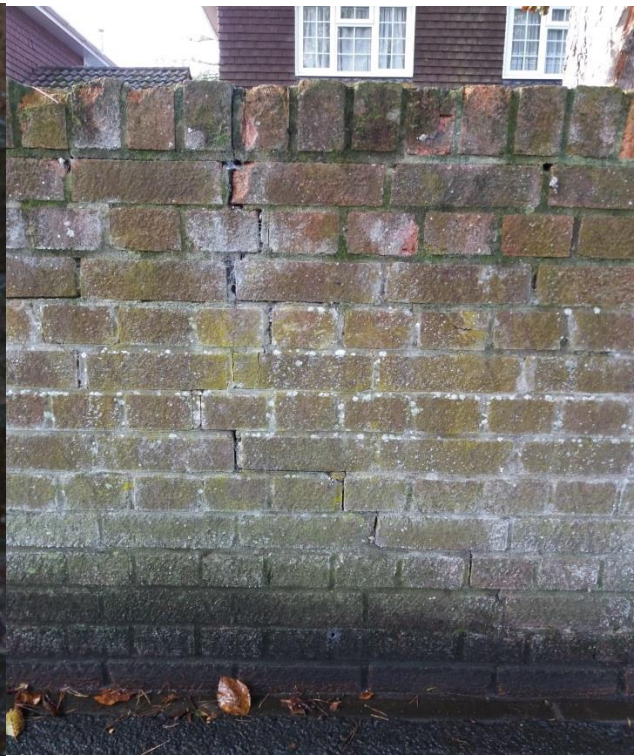
minor cracking / loose mortar
